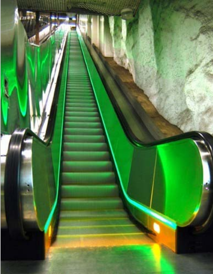
Skirt lighting reflections on stainless steel balustrade.
